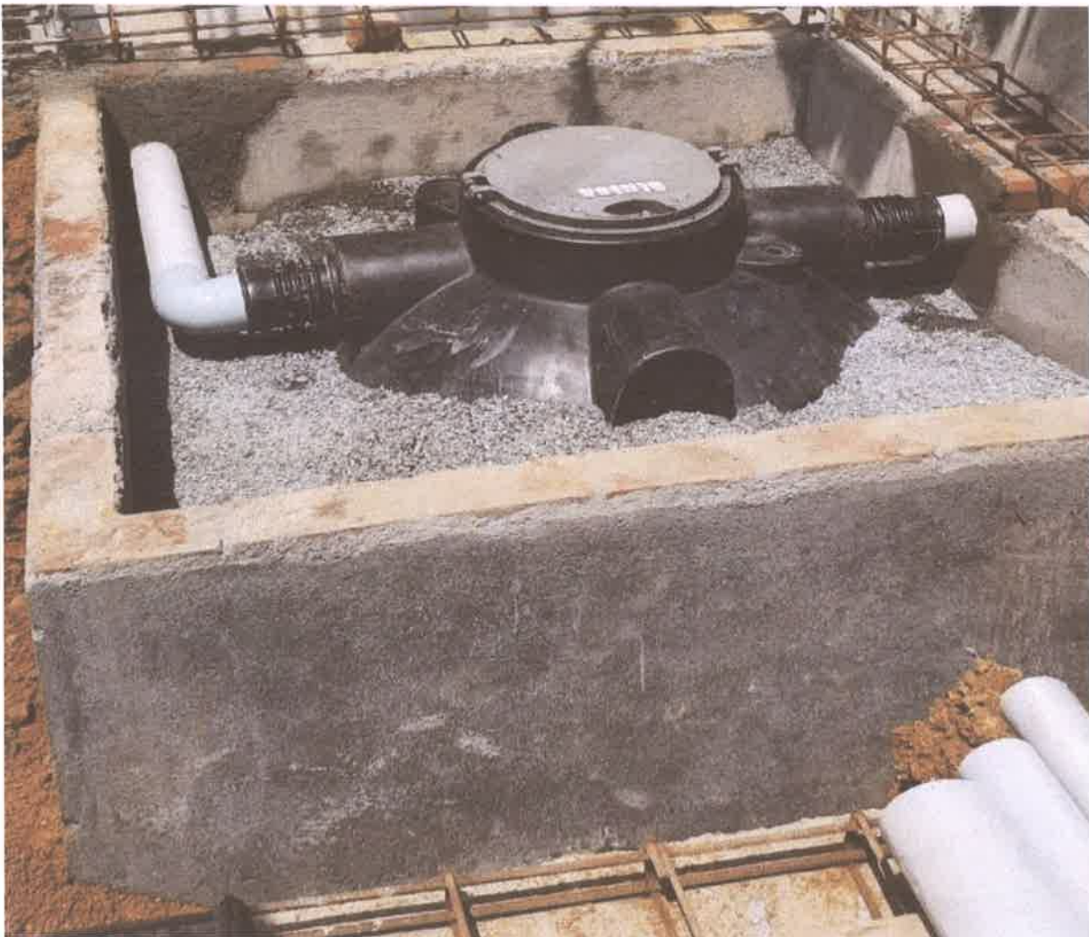
Bio Digester Septic Tank
