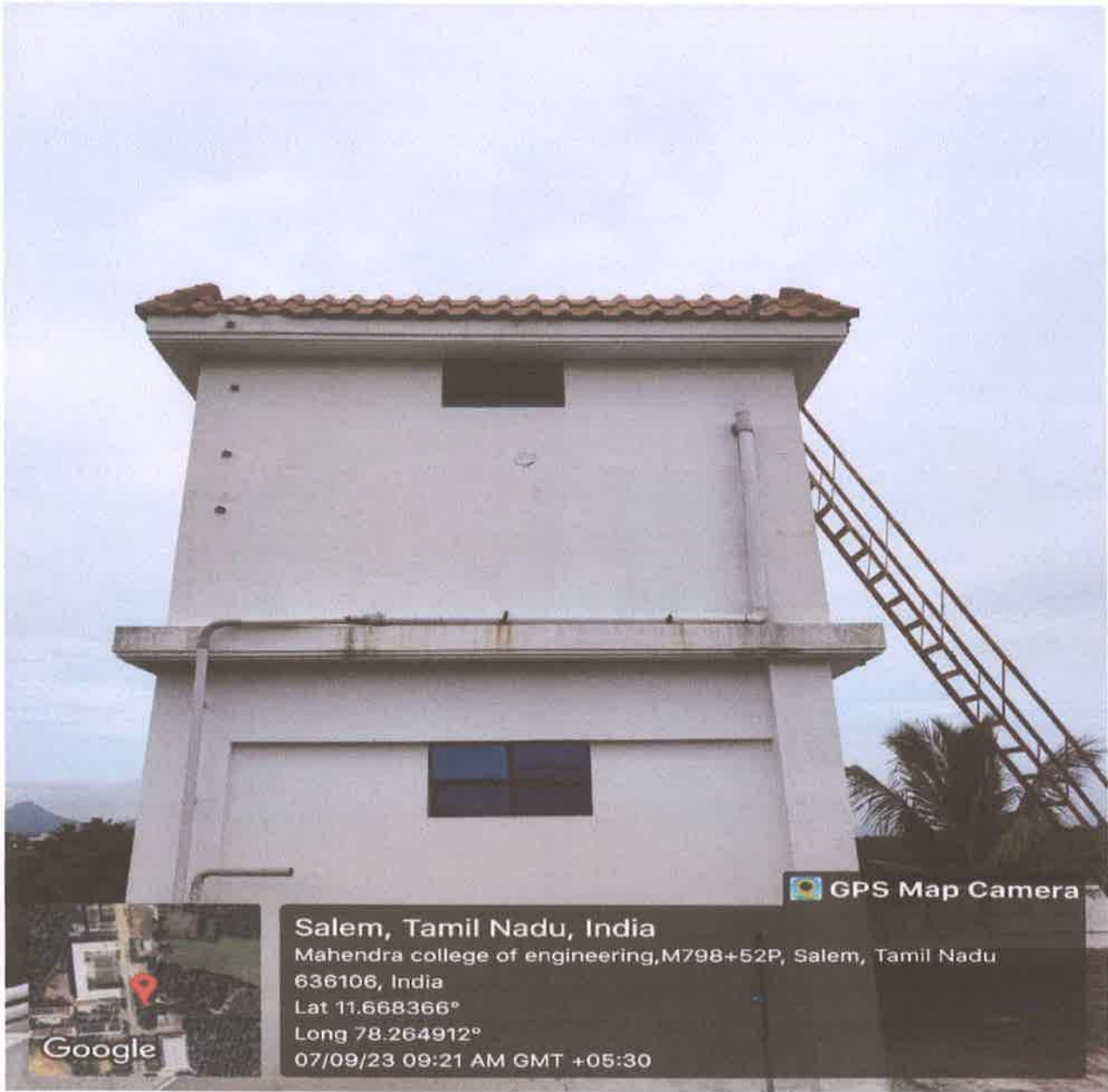
Overhead Tank with Pipeline
