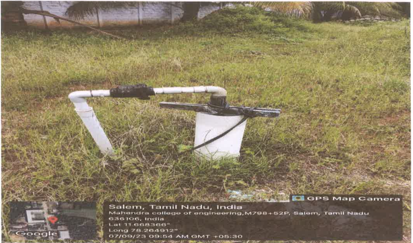
Bore Well Located Near to IT Dept
